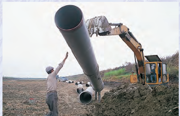
▲ 農田灌溉工程 Irrigation engineering
